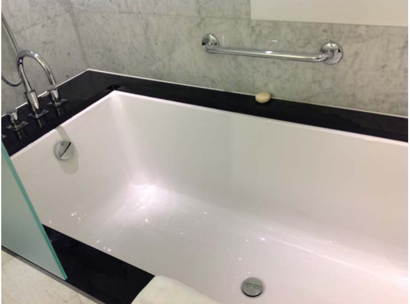
Fig 4 – Bathtub, showing the hand rail and the glass partition.
