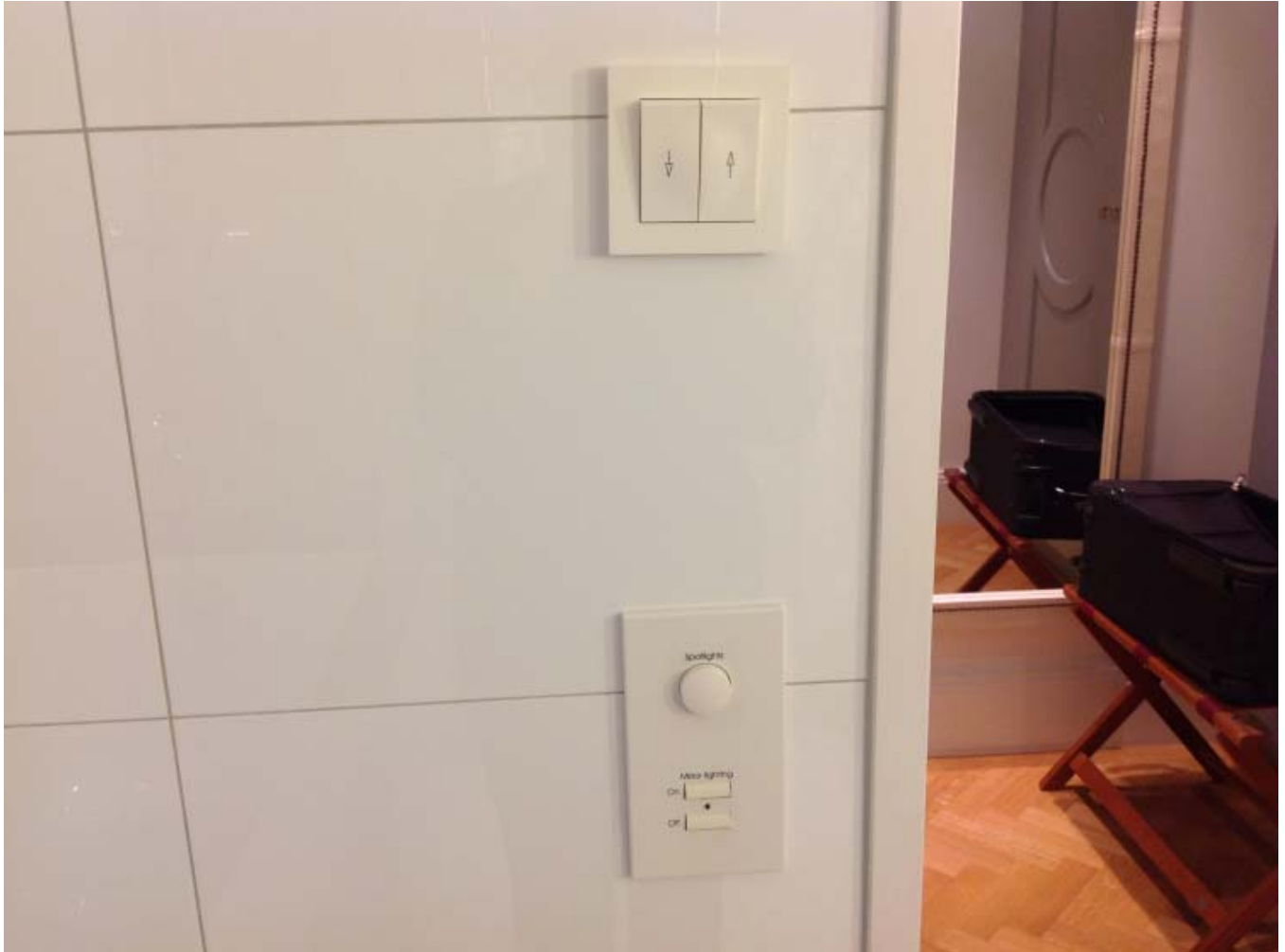
Fig 3 – Wall mounted switches in a Grand Hotel bathroom
